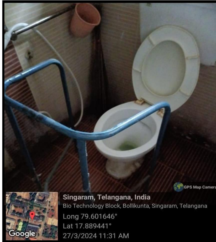
Disabled friendly Washroom
